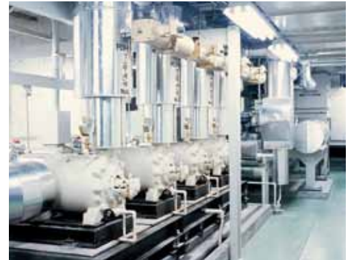
Booster pumps in water supply system of buildings
