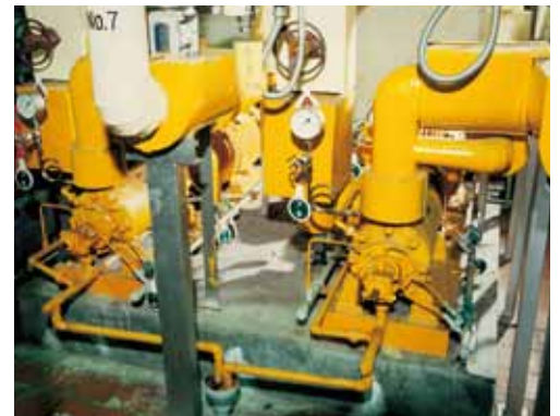
Boiler feed pumps in district heating and cooling plant
